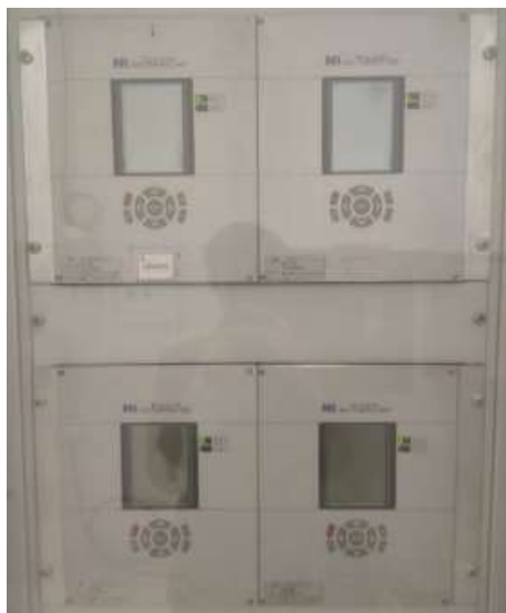
Gambar 8. Bay Control Unit (BCU)
